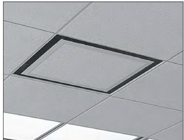
ModuFlow diffuser installed in an office environment
